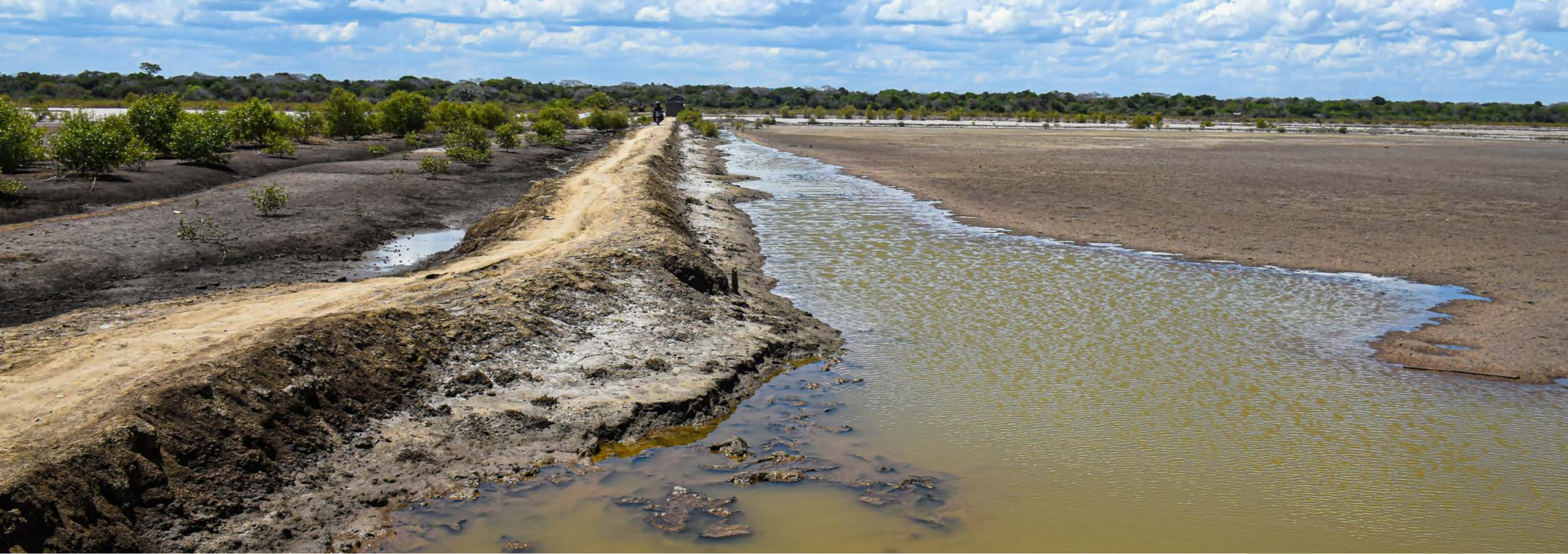
A channel dug to restore the hydrology previously disrupted by salt harvesting in Msindaji, Rufiji Delta.
