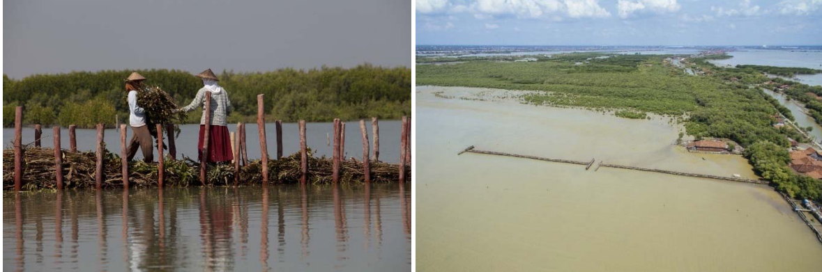
Left: Building structures to stimulate sedimentation. Right: Structures and natural mangrove - Desa Bedono (credits Nanang Sujana, Wetlands International).
